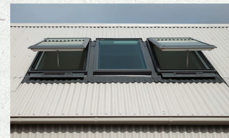
On a hot summer's day the skylights act like air chimneys, sucking the heat out.
